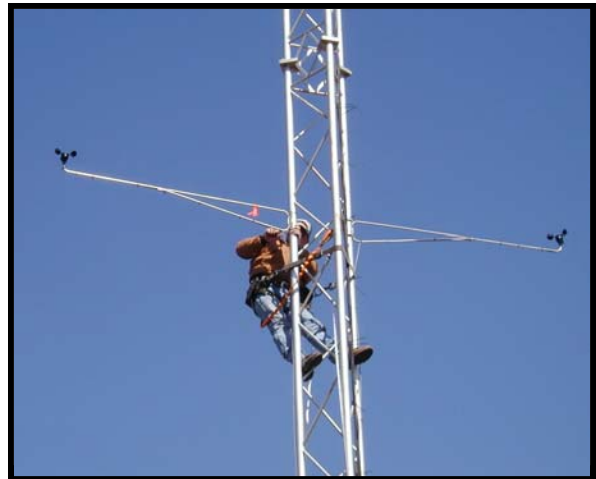
Above: Troy Choplin, tower climber for Vroom wireless, attaches the booms with wind instruments to the tower.
