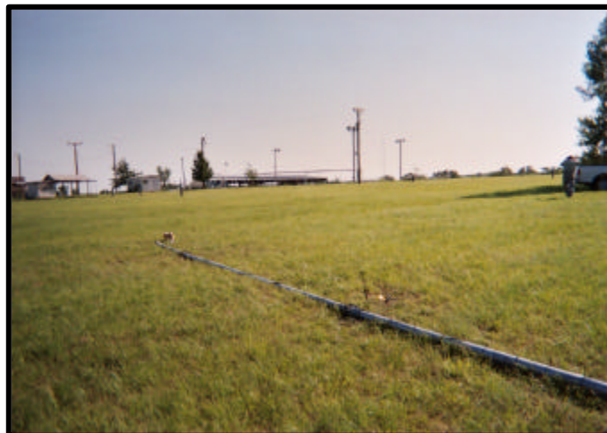
Above: The tower is laid out on the ground before being raised into position.
