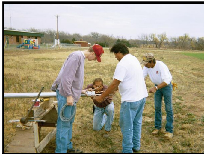
Troy Simonsen (OWPI; left side) and members of the Otoe-Missouria Tribe install wind instruments and a lightning rod atop tower.
